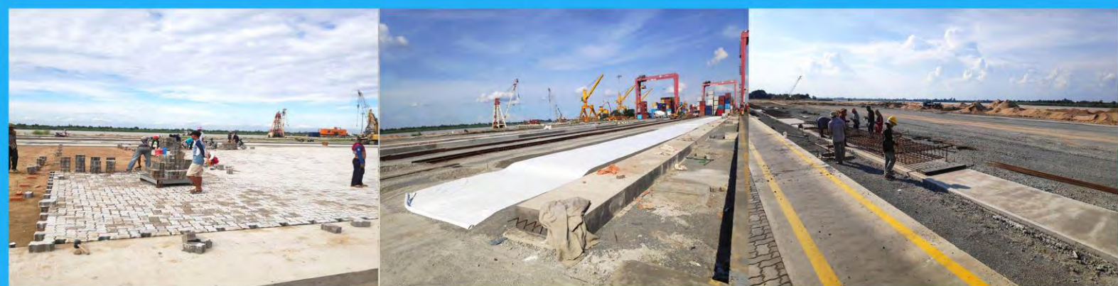
Construction of RTG lanes and concrete block yards for Phase III Expansion of the Container Yard.
